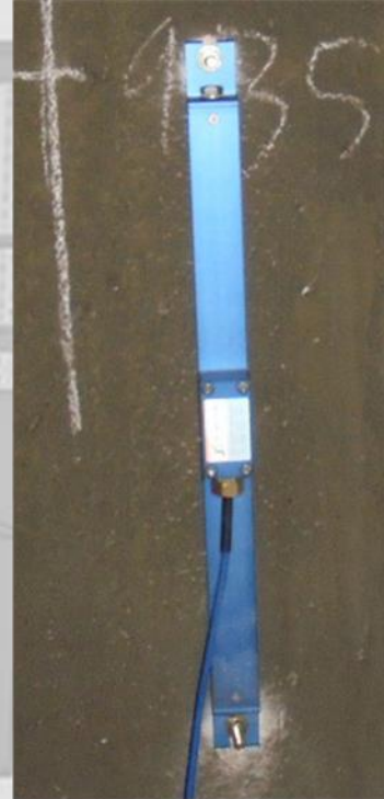
Installation Picture of EL Beam Incliner
