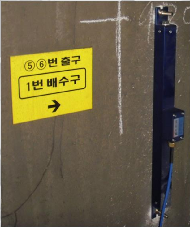
Installation Picture of EL Beam Incliner
